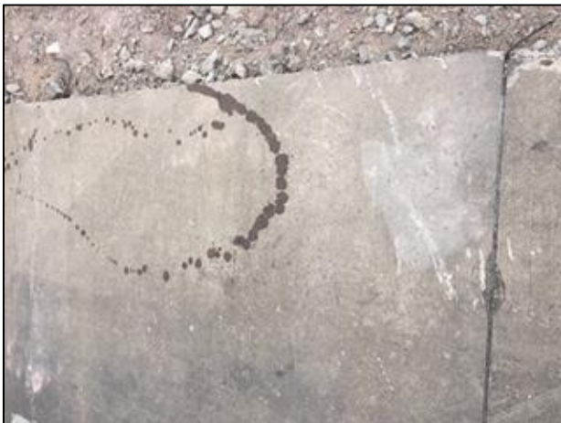
26) Minor spills observed next to the stationary plant. – September 2020
