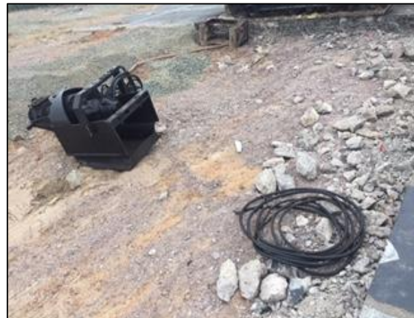
27) The oily pump was directly placed on the soil – September 2020
