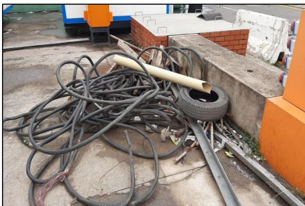
28) Waste was observed on site. –October 2020
