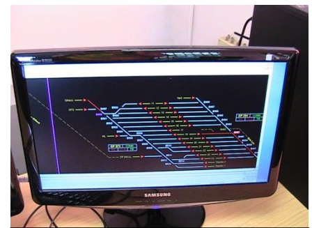
COMPUTERISED IN TOWER
